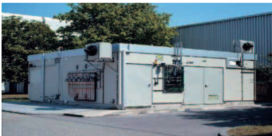
Fig. 22: Analyzer house (shelter)
