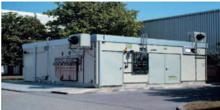
Fig. 12: Analyzer house (shelter)
