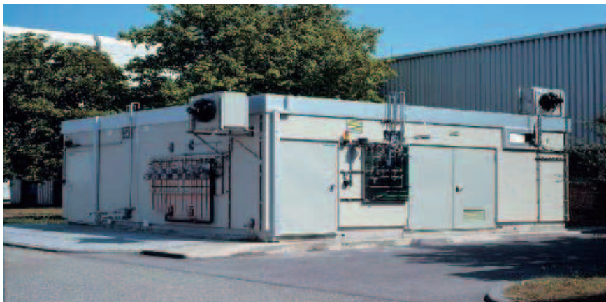
Fig. 10: Analyzer house (shelter)
