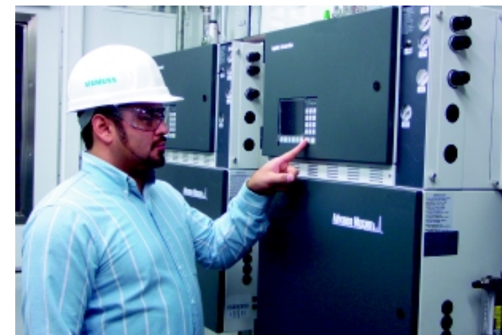
Analyzer maintenance and engineering functions can be performed at the analyzer using the MMI or via the computer workstation.
