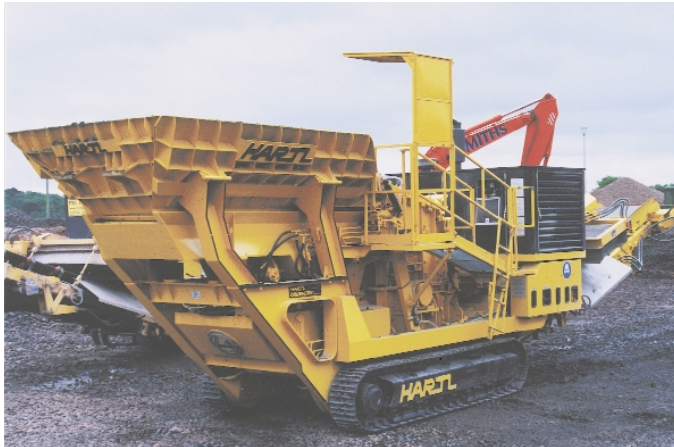
A Milltronics MSI belt scale system tallies up the daily production rates of aggregate crushed by the Hartl Crushtek International Ltd. Mobile Crusher at Severn Trent's demolished Kidderminster Wastewater Plant.
